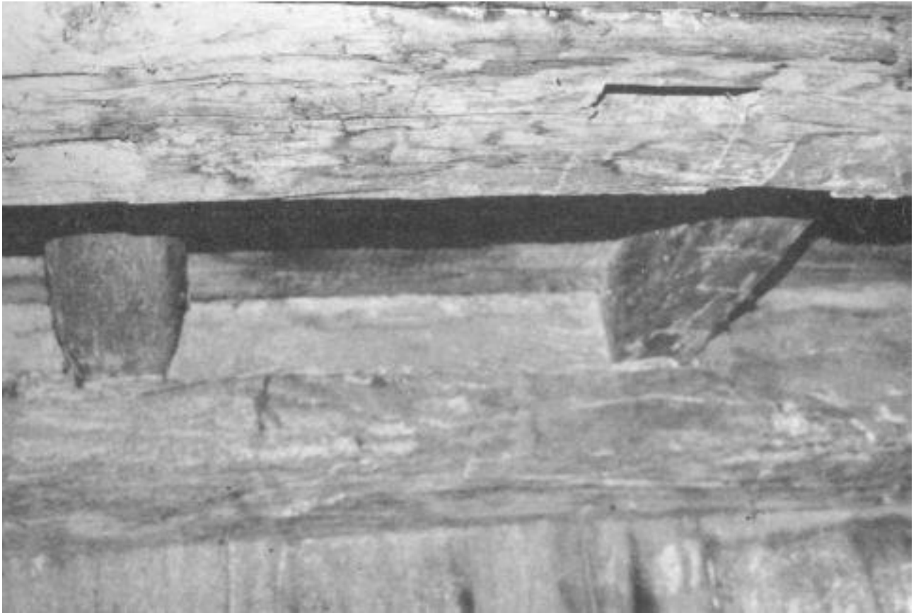
Handhewn Beams in northwest room of lower story of Higgins home, in foreground, 10 x 12 inches; others 6 x 6 inches. Photo Courtesy of Eveylyn Kreutzer.
